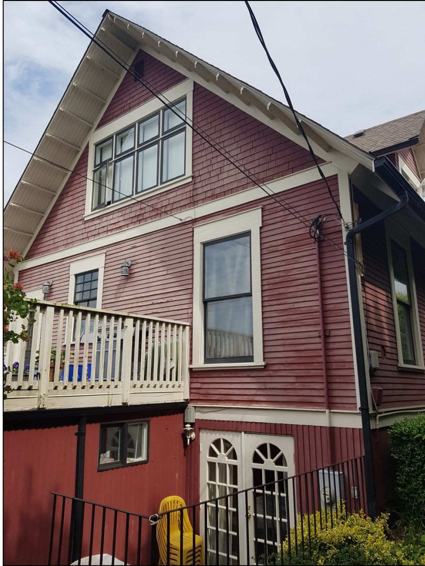
The south elevation (rear) shows evidence of failing paint due to sun exposure.
