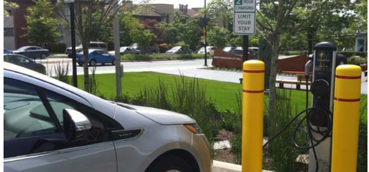
Electrical vehicle charging station
